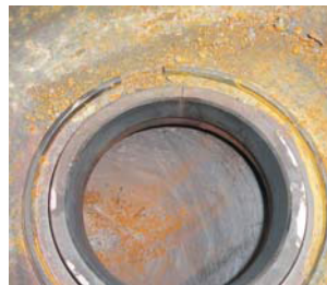
The valve seat was subject to through type cracking.
